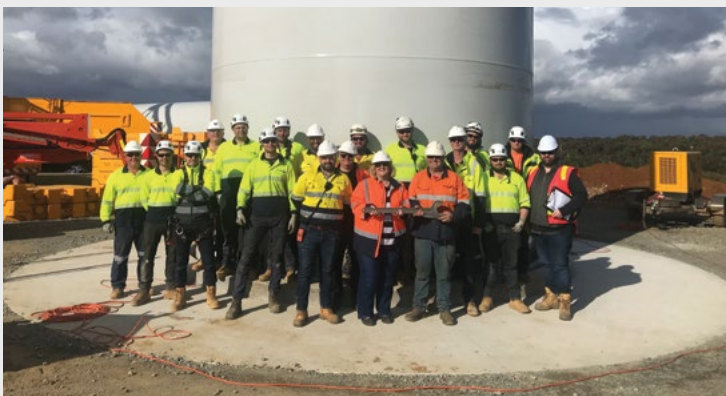
The construction team onsite with landholders Royce and Lisa Smith after the successful installation of the first tower section.
